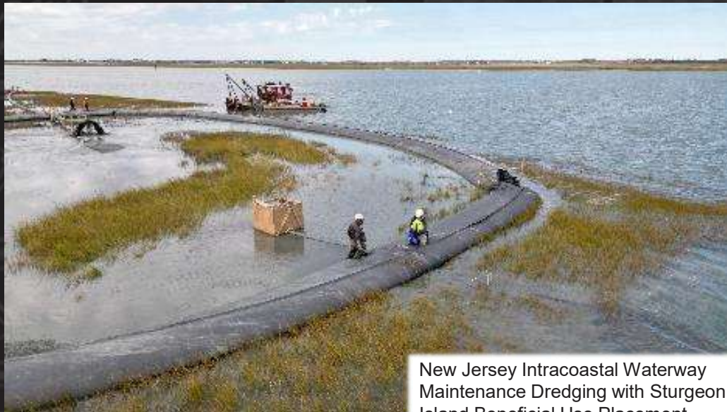
Dredge Fullerton working off of Mordecai Island, NJ for navigation and island restoration
